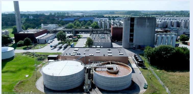
Carlsberg's Total Water Management plant at its Danish brewery
